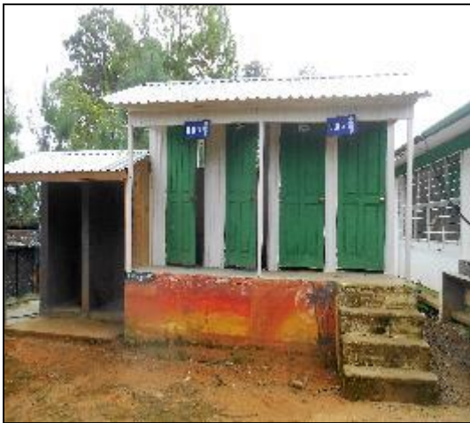
Figura36. Baños secos bachilleres
