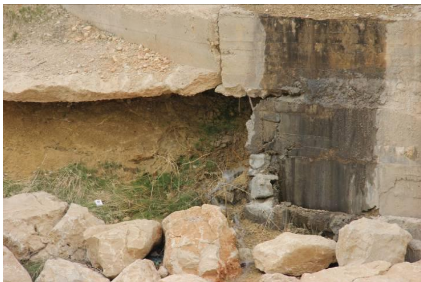
Fig. 1. b) Piping hole and seeping flow between abutment and concrete body at downstream
