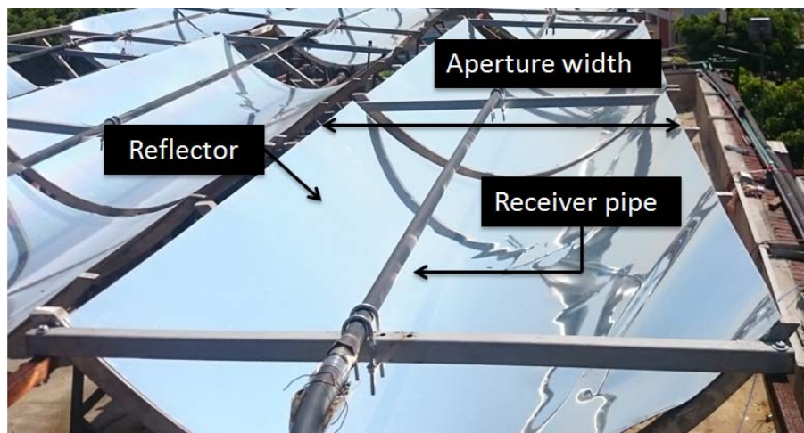
Figure 5. Photograph of the parabolic trough collector used in this work.
